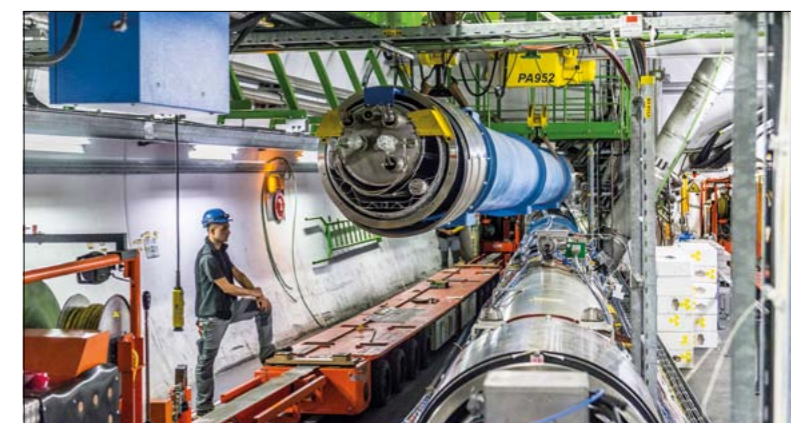
(Top left) A replacement magnet is lowered slowly down the special access shaft to the transfer tunnel to the LHC. (Top right) The specialized trailer with one of the replacement magnets follows the white line en route to its final location in the LHC tunnel. (Above) A magnet is lifted off the trailer at its final location for installation in the LHC's 27 km ring.
